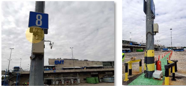
Figure 118: Madrid Mega pilot site: RSU installation, at Carabanchel
